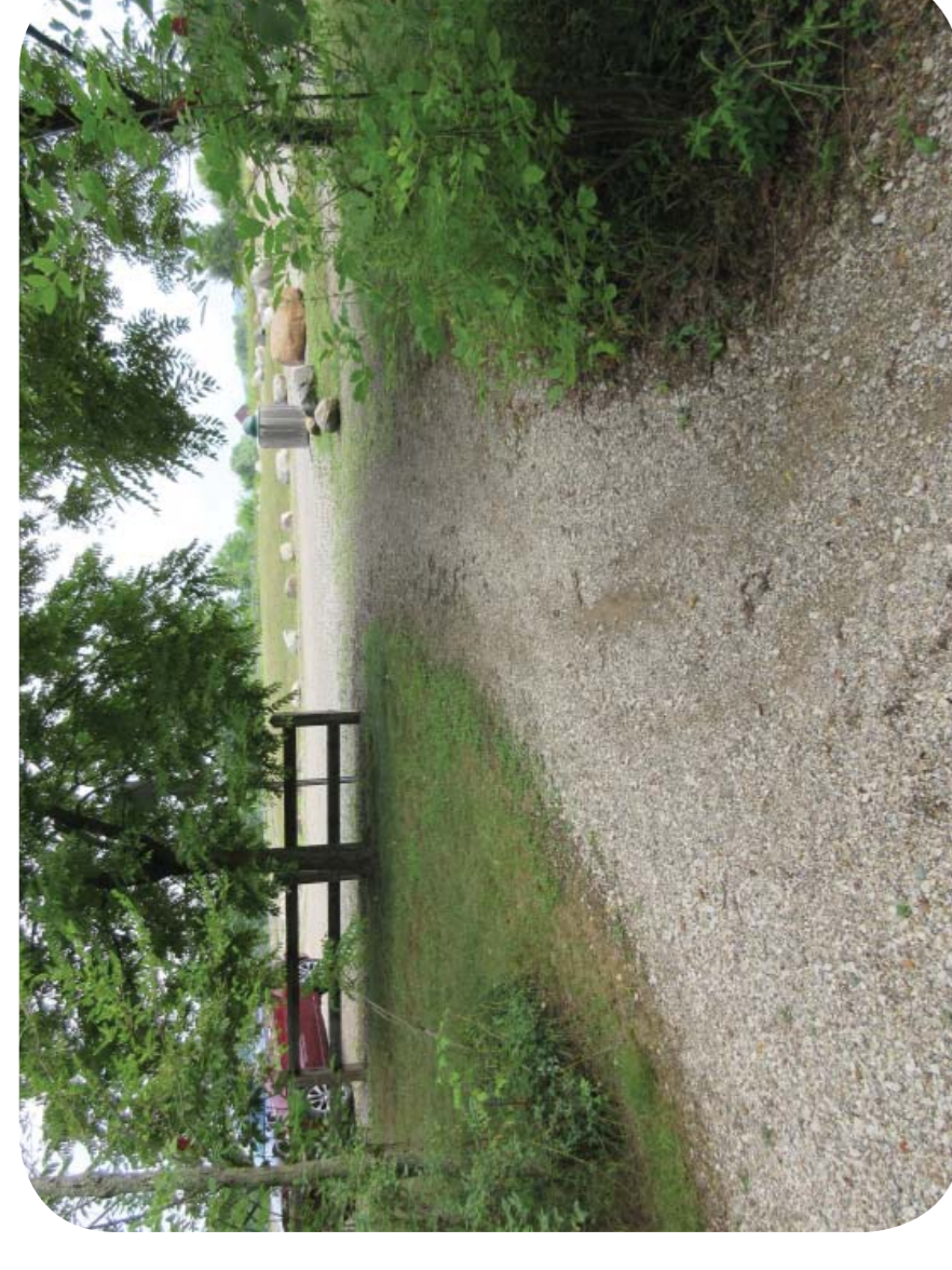
ACCESSIBLE ROUTE DOES NOT MEET ADA STANDARDS FOR MATERIALS AND GRADING.
