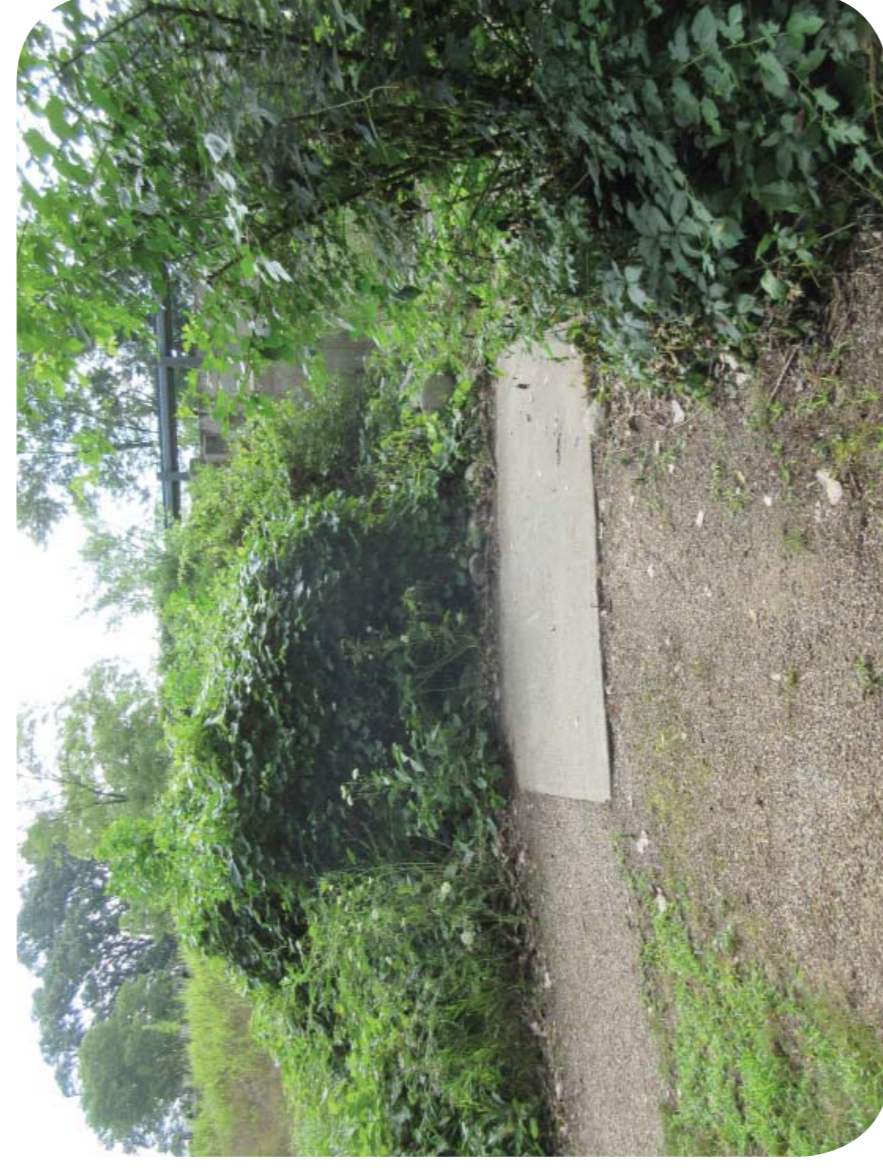
CRUSHED GRAVEL PATH CONNECTION TO CONCRETE SIDEWALK DOES NOT MEET ADA STANDARDS.
